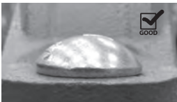
GOOD BOLT ENGAGEMENT (OVAL NECK OF EACH BOLT IS SEATED PROPERLY IN THE BOLT HOLE)
