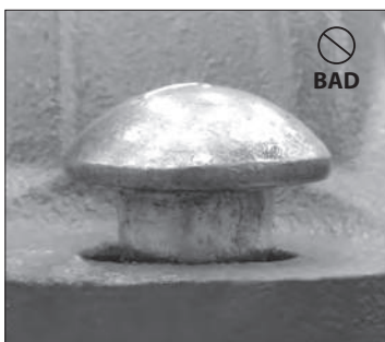
BAD BOLT ENGAGEMENT (OVAL NECK IS NOT SEATED PROPERLY IN THE BOLT HOLE)
