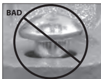
OVAL NECK OF BOLT NOT SEATED PROPERLY
