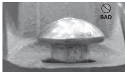
BAD BOLT ENGAGEMENT (OVAL NECK OF BOLT IS NOT SEATED PROPERLY IN THE BOLT HOLE)
